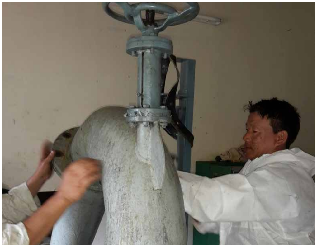
Fig. 23 DGPC's O&M Personnel Supports Annual Maintenance Works at Sengor Micro Hydel Plant Since 2012
