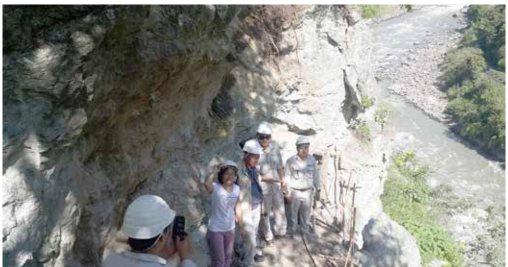
Fig. 10 Right Bank Drift Portal, Dam Axis Upper Drift of Dorjilung (Kuri I) Hydropower Project
